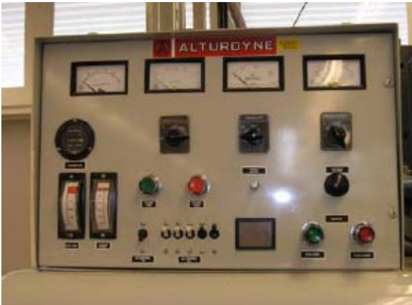
Figure #5 Engine Control Panel
