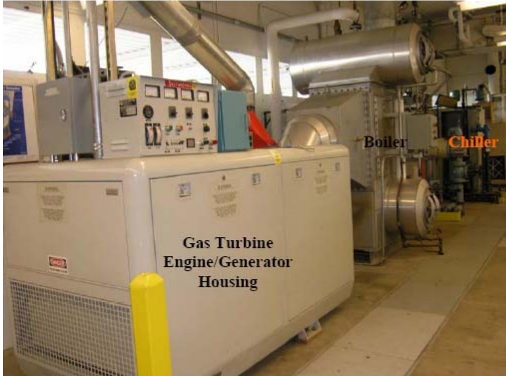
Figure #3 Cogeneration System
